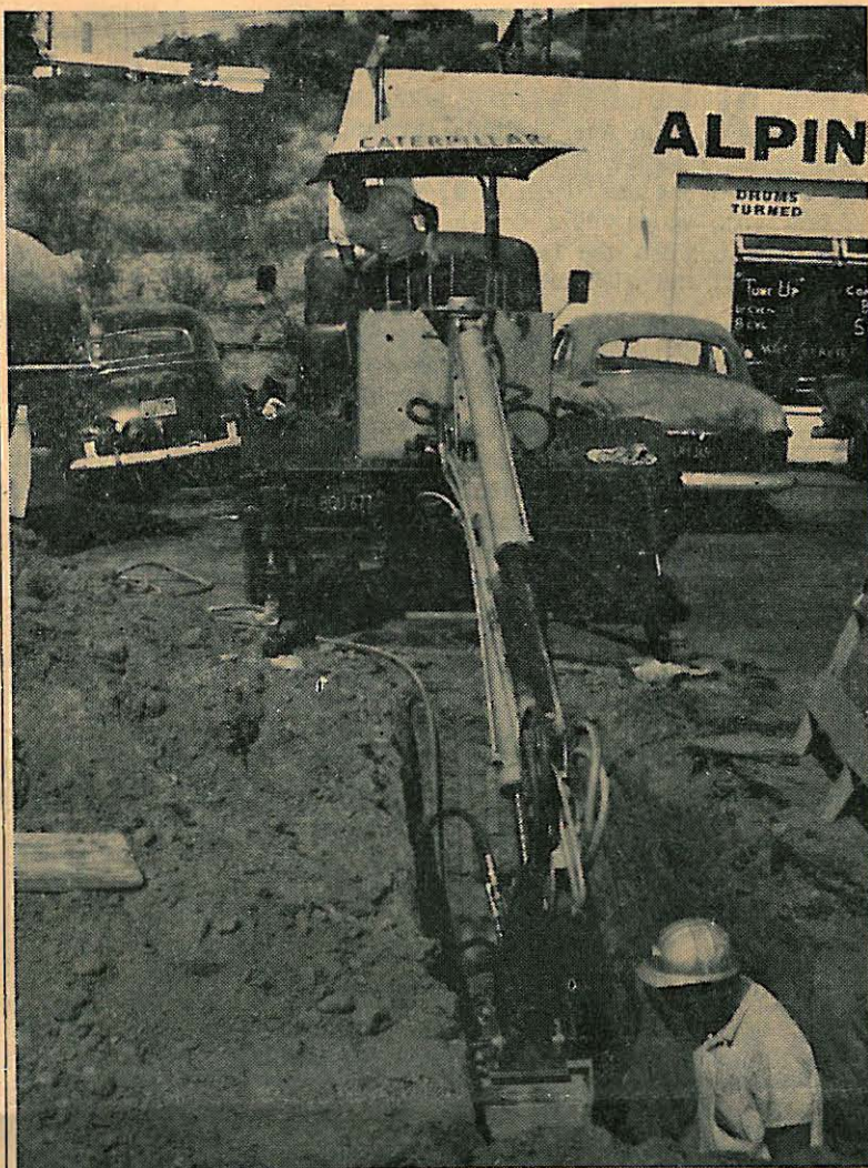
Contractor's equipment and crew "jacking" pipe under pavement on Highway 80 in front of Alpine Auto Parts being installed by Rio San Diego as a portion of the water line to serve the Alpine Fire Station and the Alpine Elementary School.
